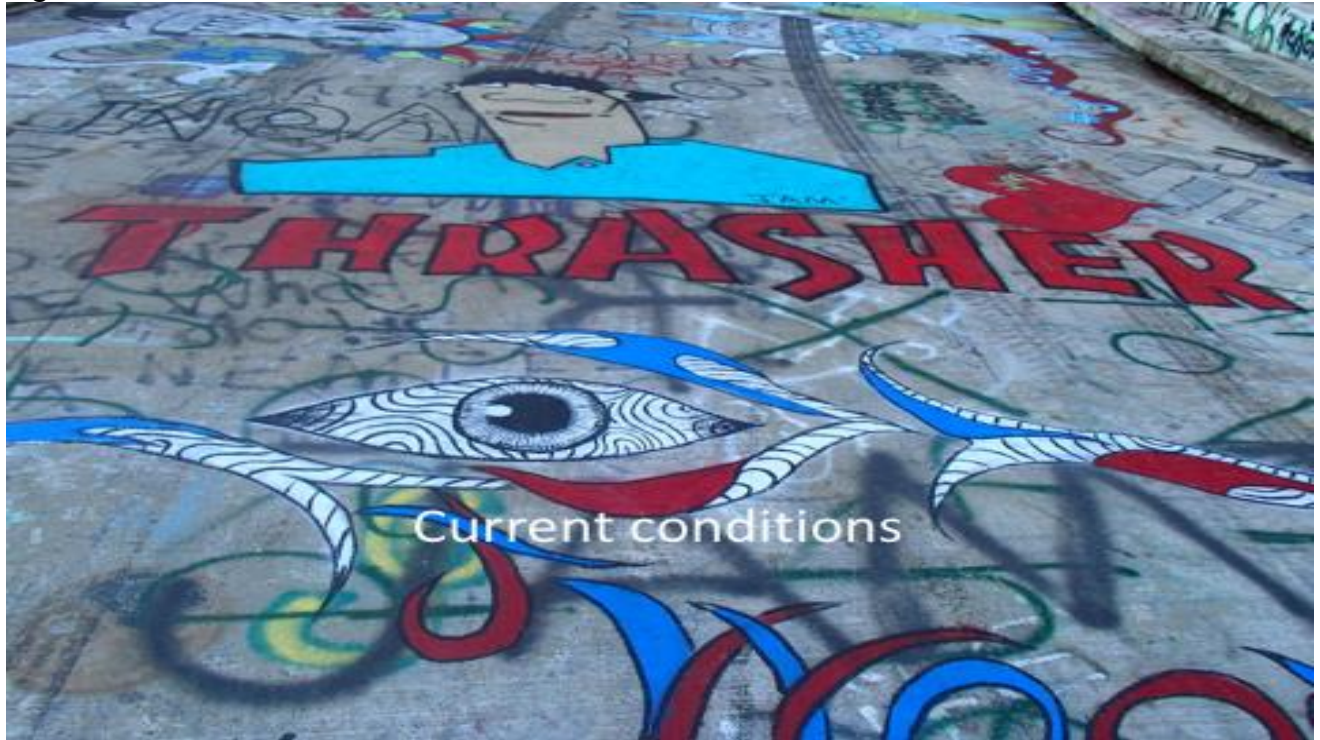
Figure 3. Shows vandalism of area.
