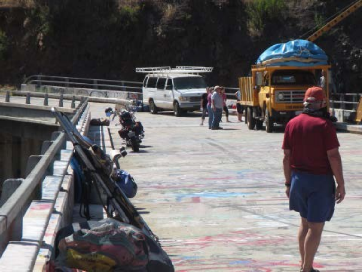
Figure 3. Demonstrates pedestrian safety concerns on the bridge.
