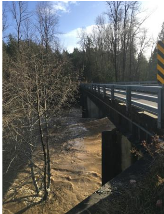
The tank crossing bridge is an undeveloped access point on JBLM that requires an access pass. Photo: Morgan Greene
